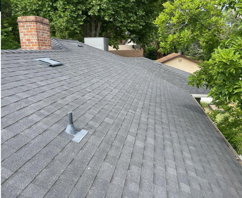
Attic ventilation with O'hagin Vents - will help keep the house cool
