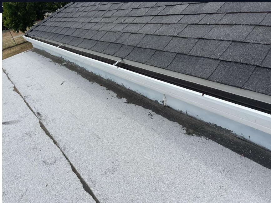
Roof to Wall sealed with mastic - roofing sealant. This is a temporary repair.
