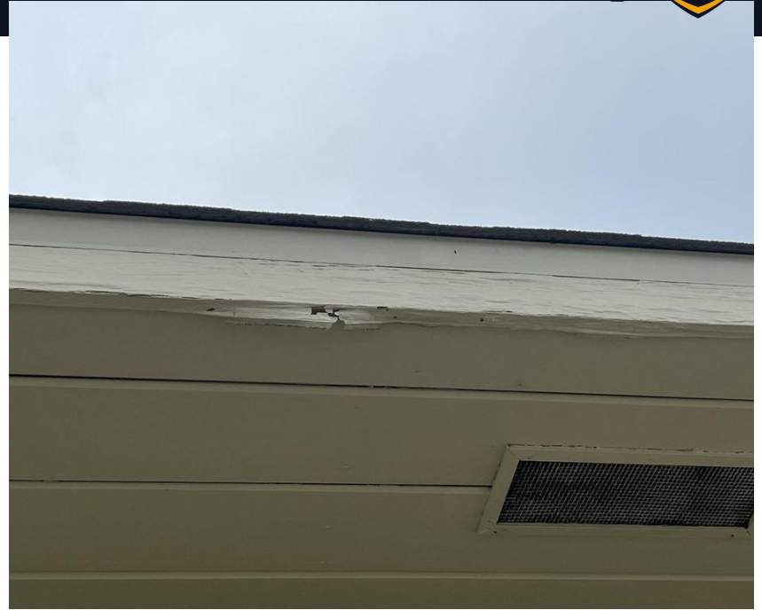
Slight dry rot damage to fascia boards, most likely from previous roof system.
